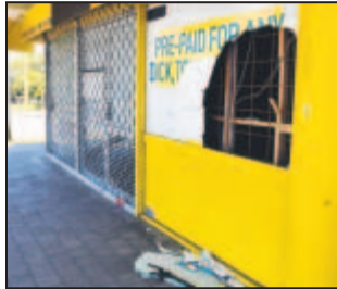
ABANDONED: Dilapidated shops at Horton Pde.
